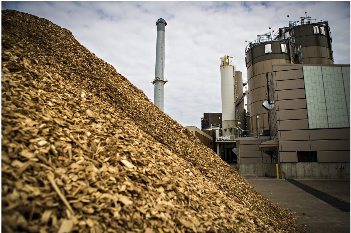
Photo of biomass boiler using grass and wood chips. Photo courtesy of Kyle Spradley, Curators of the University of Missouri, 2014. Info on the rights reserved: http://creativecommons.org/licenses/by-nc/4.0/
