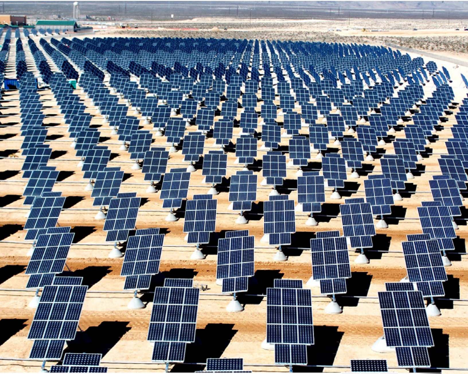
Nellis Solar Power Plant located within Nellis Air Force Base, northeast of Las Vegas, Nevada, United States. The power plant occupies 140 acres, contains about 70,000 solar panels and generates 14 megawatts of solar power for the base.
