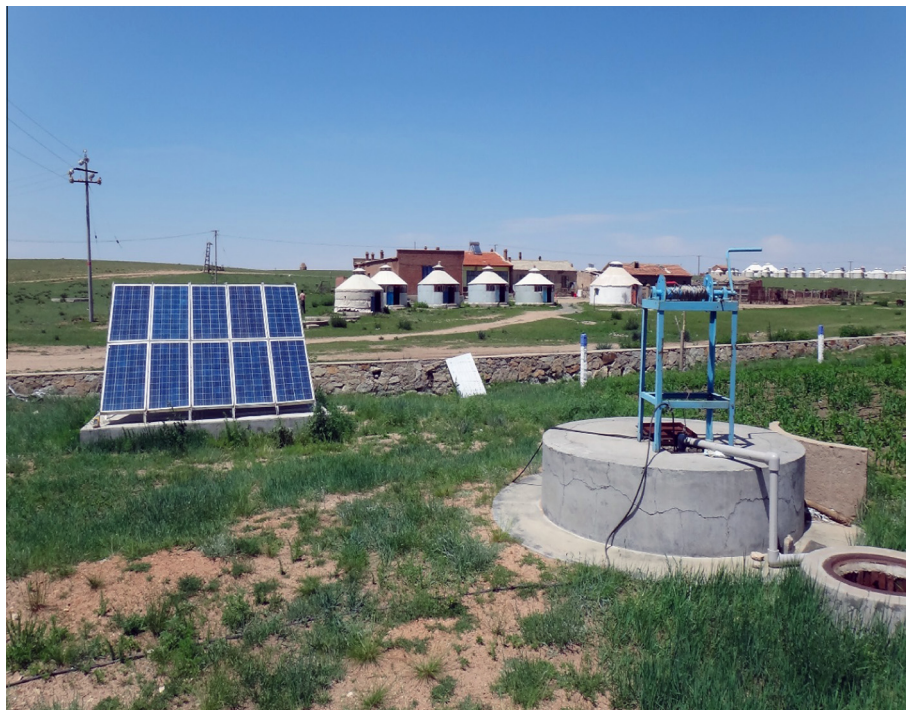
Fig. 4. PVWP system for irrigation installed in Xilamuren, Inner Mongolia (the PV array is installed nearby the available electric grid).
