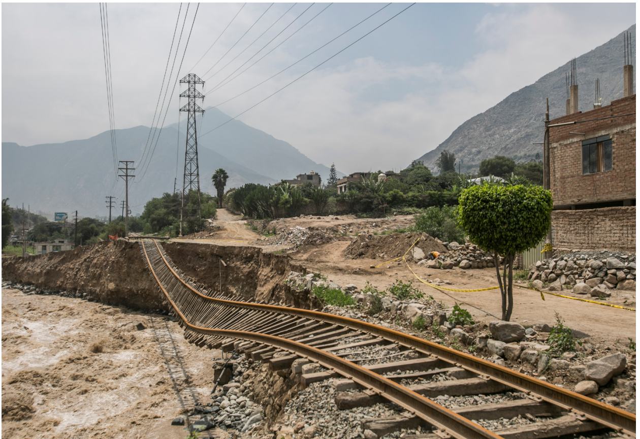
Photo 5: Railway and road damage from erosion along the Rimac River in 2017.
