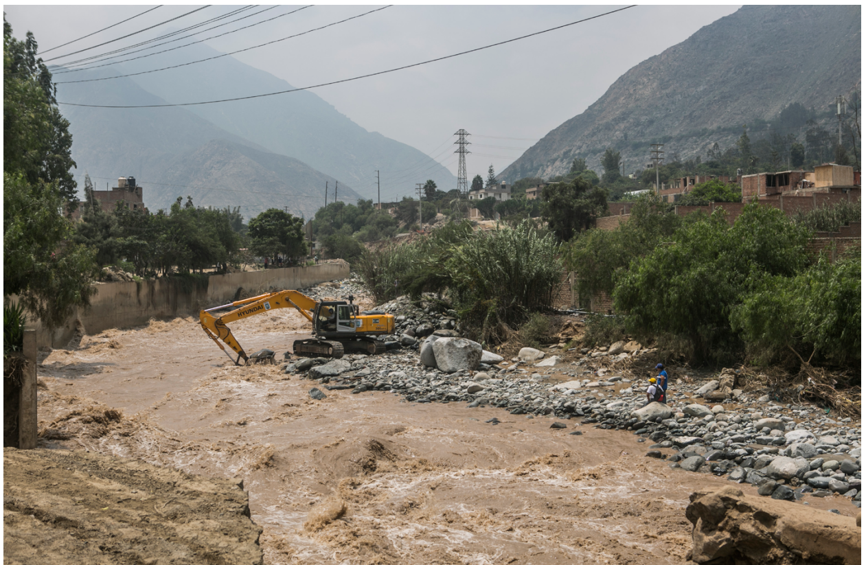
Photo 6: Ongoing efforts to open the channel of the Rimac River as flooding impacts intensified during early 2017.
