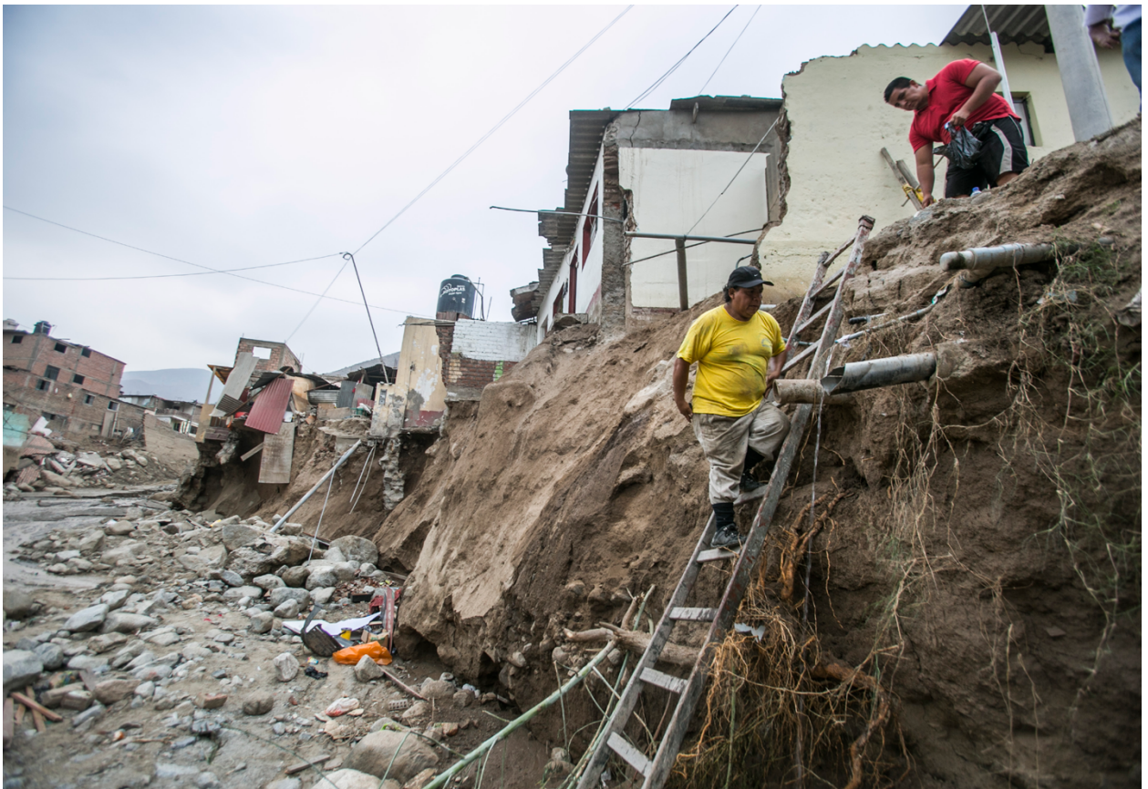
Photo 4: Water and sewage lines exposed by flash-flooding-induced erosion in early 2017.
