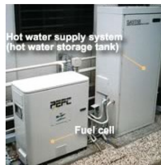
(Residential use-fuel cell system installation test: http://www.gas.or.jp/gasfacts_e/12_e.html )
