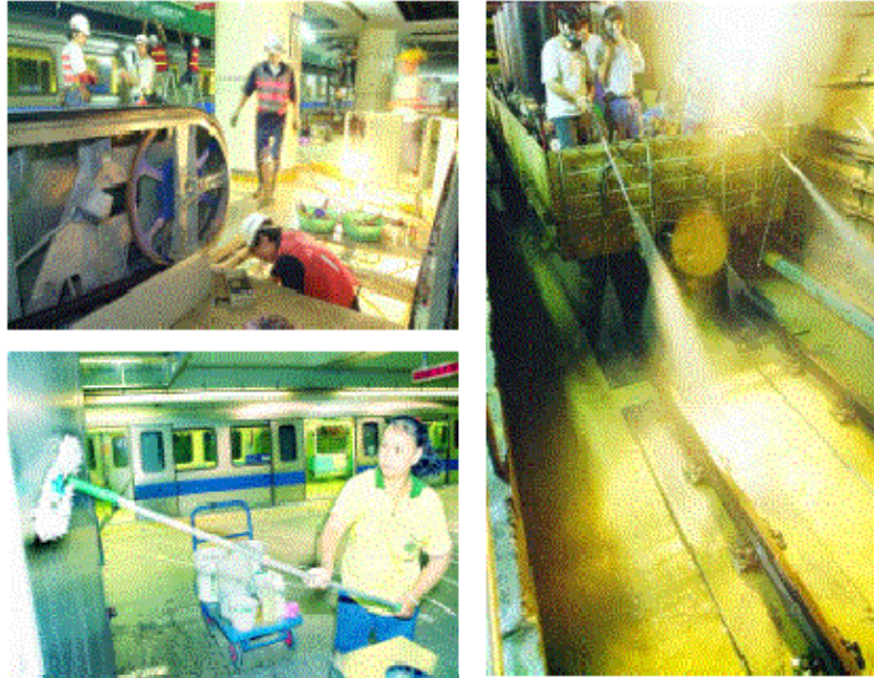
Figure 4.2: Cleanup and repair work on the MRT Photo credits: George Tsorng, Taipei Times
